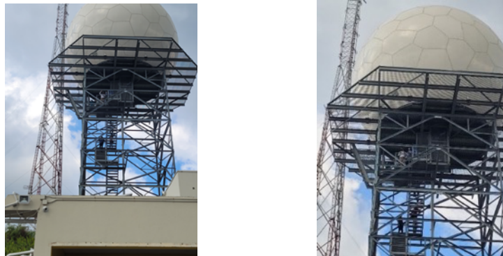
Figure 7. Jamaica's radar radome and tower.
